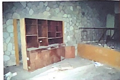
Interior of an abandoned house. It was a beautiful house situated on a hillside opposite the volcano. On one side was a lovely view of Plymouth. On the other side a view of the Chance's Peak volcano also known as Soufriere.
